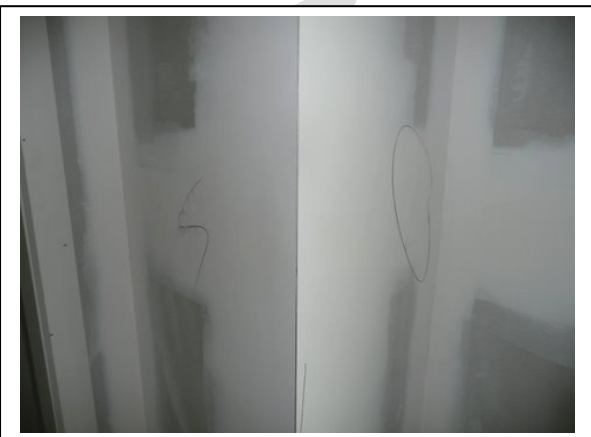
Plaster marked up to show defects
