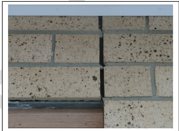
Expansion joints to bricks not filled
